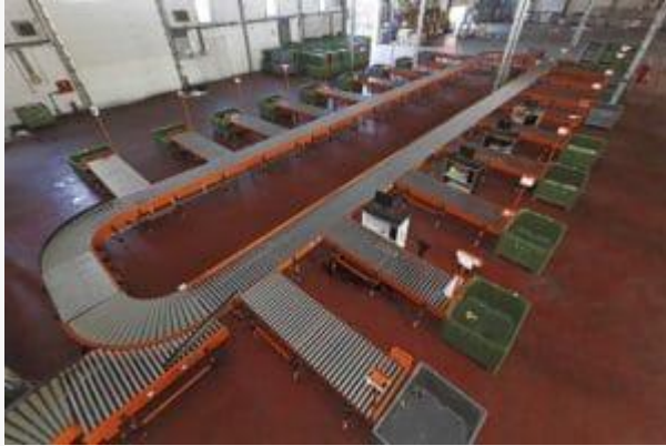
Arm/pusher style sorter conveyor system
