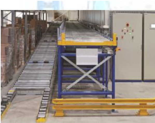
Gravity Conveyor System
