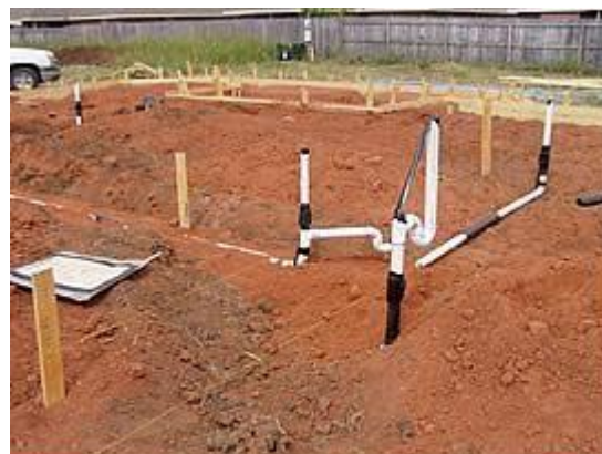
This plumbing will be beneath and poking through a floor slab.
