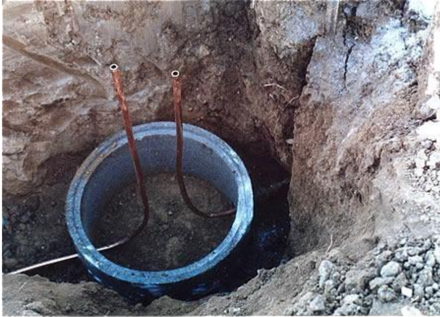
This is a water meter pit. One copper pipe is coming from the city supply line in the street. The other pipe will supply the new home with water. A meter to supply billing information to the city will connect the two.
