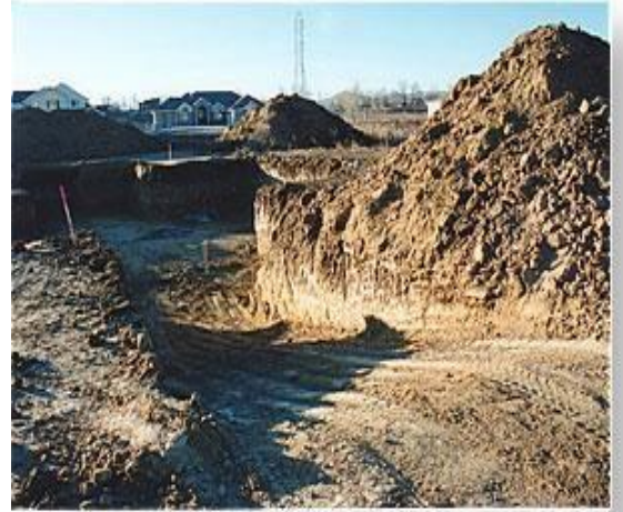
Excavation for a basement home. Notice the temporary ramp that has been constructed so that the dozer can get down in the hole.
