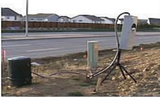
Temporary Electric "Saw Service"
