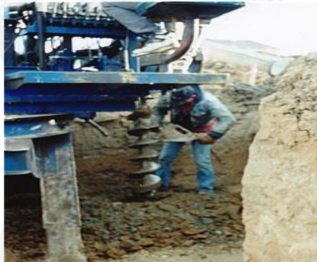
This sub is drilling a hole to pour a "caisson" - a special type of footing used in areas with highly active soils.
